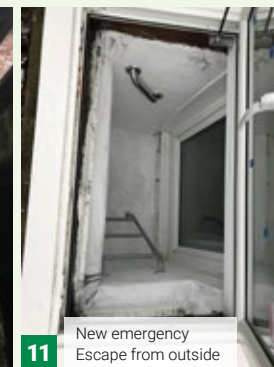
11 New emergency escape from outside
